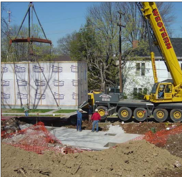
This picture shows the EFI provided crane contractor off-loading the station from the EFI delivery truck using EFI provided rigging and slings.
