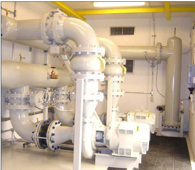
This picture shows the internal mechanical and plumbing system for the two (2) – 125 horsepower, end suction centrifugal pumps with piping, valves and support structure. The building built by EFI supports a 2000 pound capacity bridge crane for use in safely servicing pumps and valves as is required.
