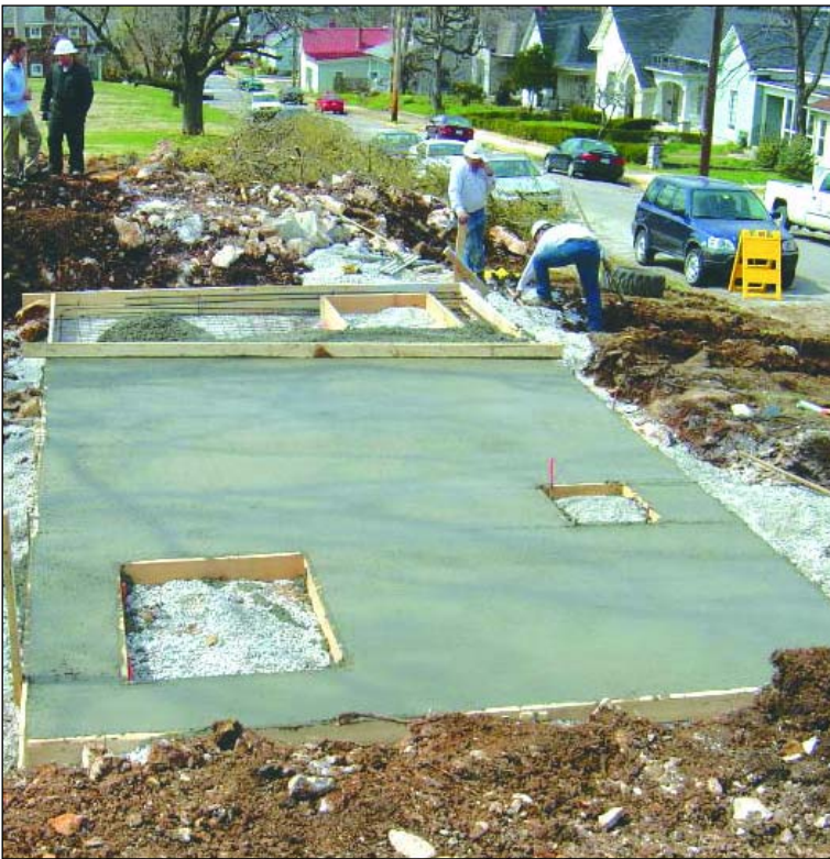
In this picture the slab-on-grade foundation is being poured. EFI provided the foundation design based on BGMU provided soil condition data.
