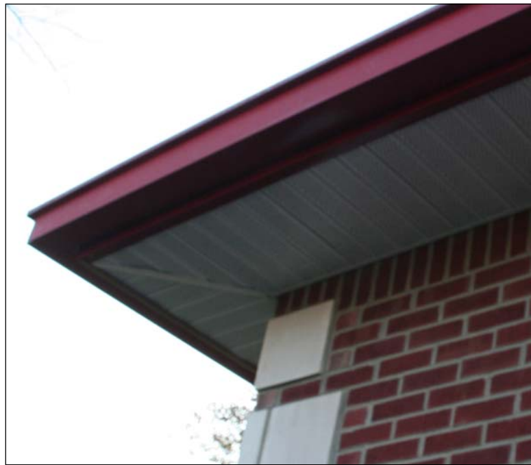
This picture shows one corner of the underside of the aluminum, standing seam metal roof, eve caps and the soffit work. The roof trusses and sheathing and the cover materials were provided and installed by a local roofing contractor as a sub-contractor to EFI.
