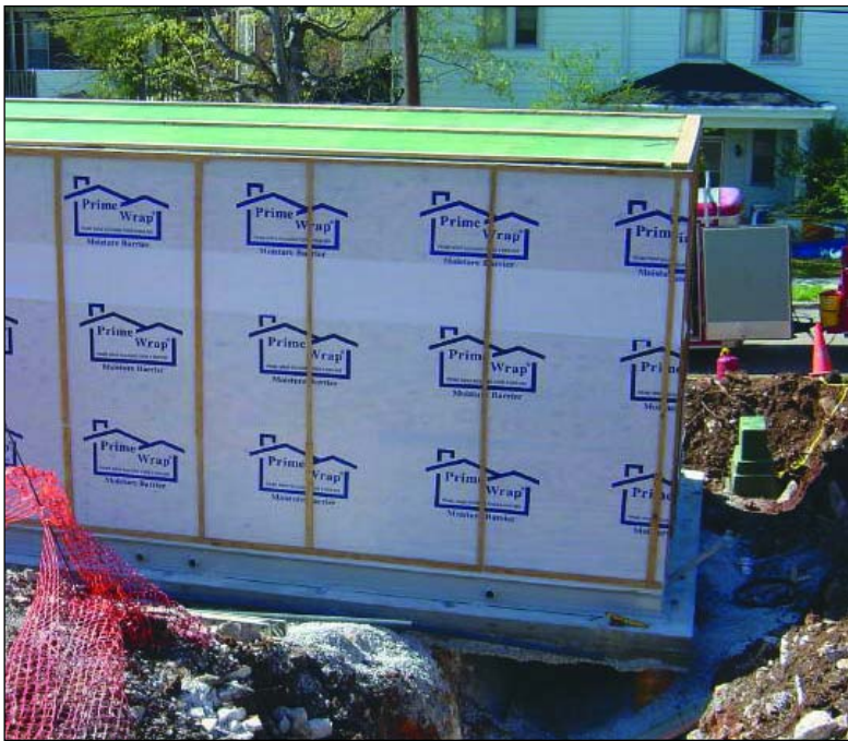
This picture shows the EFI station set in place but without the roof trusses and the exterior masonry. The truss sill boards were placed at the Factory so as to be properly anchored into the roof joist system.
