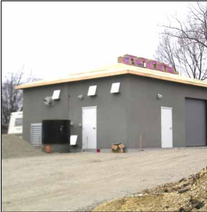
Here shown is the trussed roof structure spanning across both flat roofs of the side-by-side building halves with plywood sheathing over the trusses and ready for shingles.
