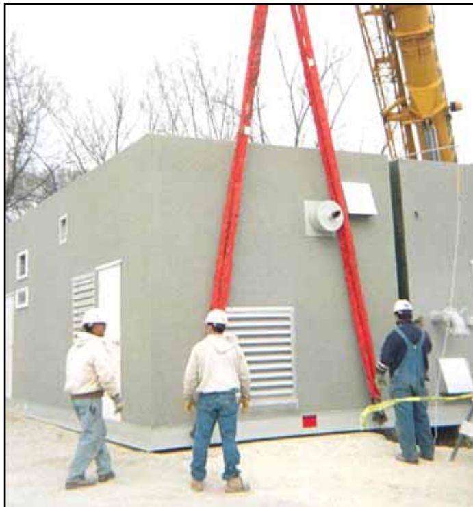
Here shown is the western half being moved into its final location by “walking” it into place using the end lifting points.
