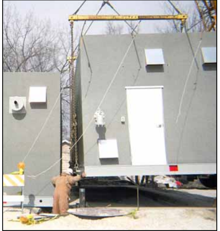
Here shown is the eastern half of the building being guided into its final location.
