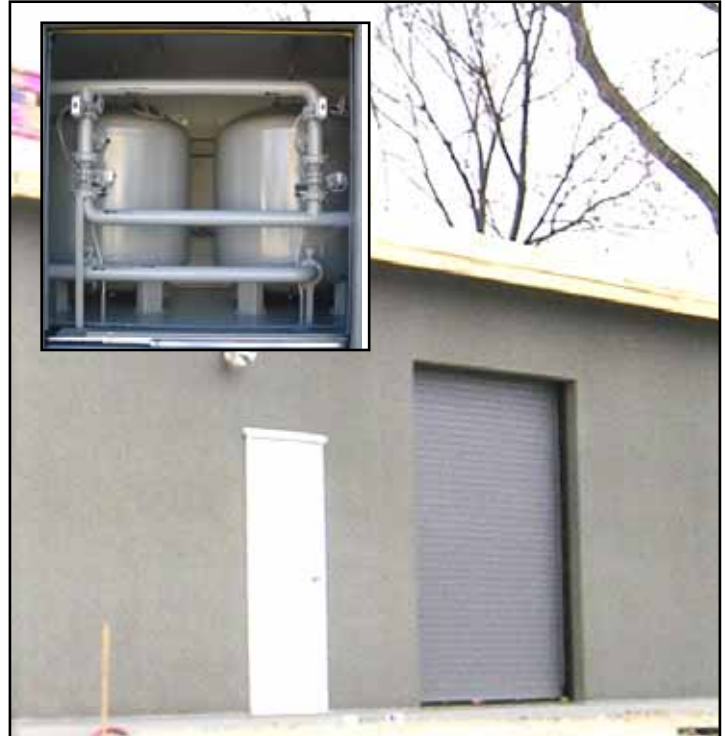
Here shown is the the man-door and overhead door in the eastern building half for access to the 4500 gallon detention tank and two 7 foot diameter pressure filter tanks with filter controls.
