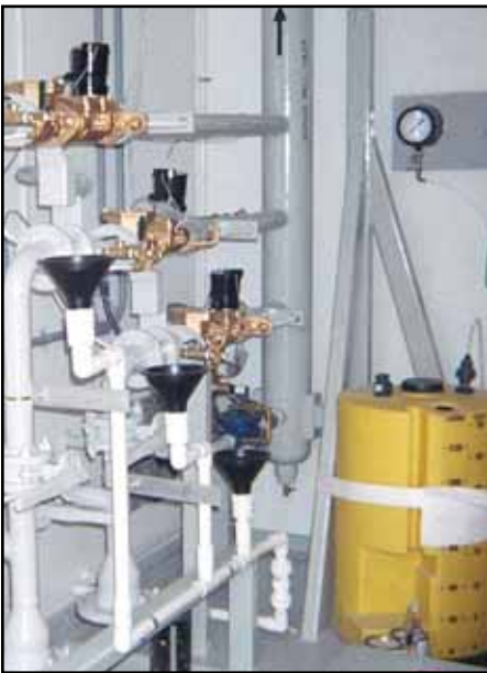
Here shown is the pre-treatment chlorine feed room with piping from each of the three wells coming into the station from underground. The three well lines have chlorine injection points and are connected to a common header with an air release valve and a flanged connection point for a pipe to connect to the other side of the station taking water to the detention tank.
